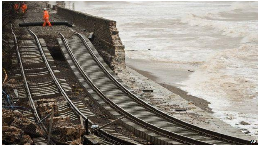
Figure 2: Section of rail track dangles over the sea after the wall collapsed at Dawlish, Devon. (Source: BBC.)
