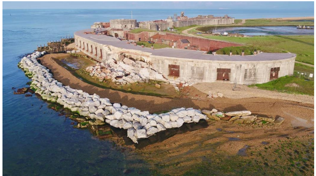
Figure 4. Hurst Castle showing collapsed portion of east wing and extent of stabilisation measures (copyright English Heritage).
